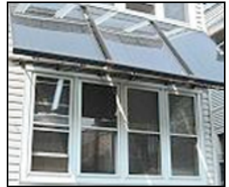
Kathy Cummings' South Side three-flat uses both solar electric and solar hot water.
