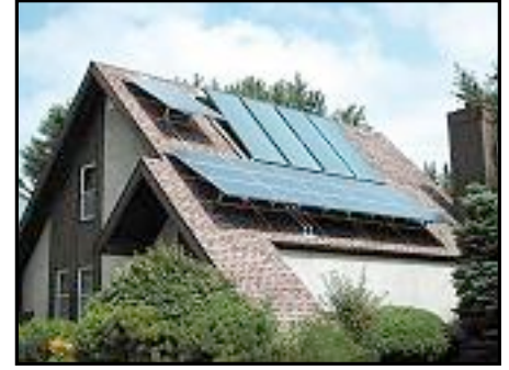
Jim and Kath Camasto's Naperville house will be on the Solar Tour Saturday. A solar thermal system, along with a high-efficiency furnace, cuts natural gas use 50 percent.
